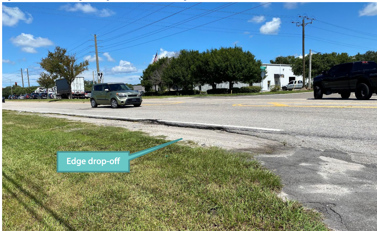
Figure 20: Erosion Along the Edge of Pavement (looking north)
